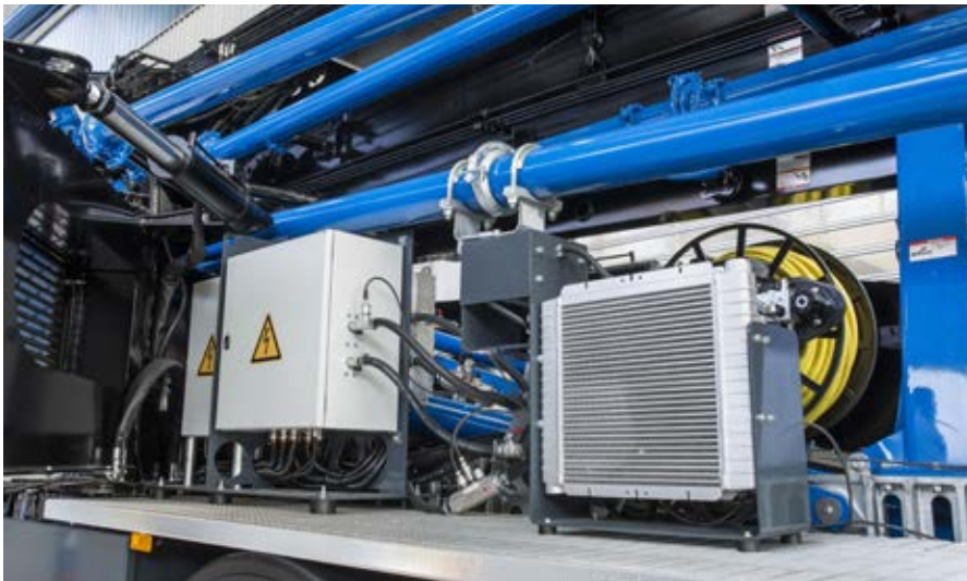
Small switch cabinet and compact liquid cooler
